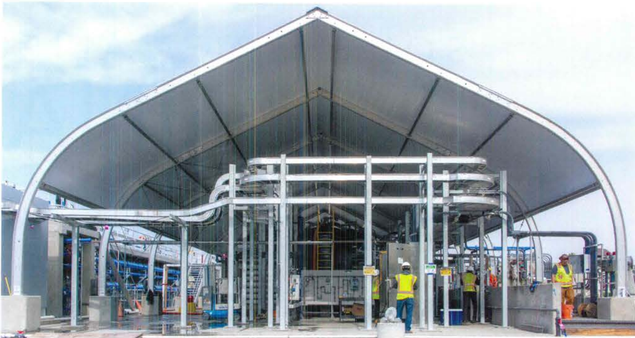
The Regional Recycled Water Advanced Purification Plant at the Sanitation Districts' Joint Water Pollution Control Center in Carson is now up and running. The plant, a joint project of the Sanitation Districts and the Metropolitan Water District, purifies about 500,000 gallons of treated water per day. Currently, treated water is discharged to the ocean. Photos courtesy of the Metropolitan Water District of Southern California
